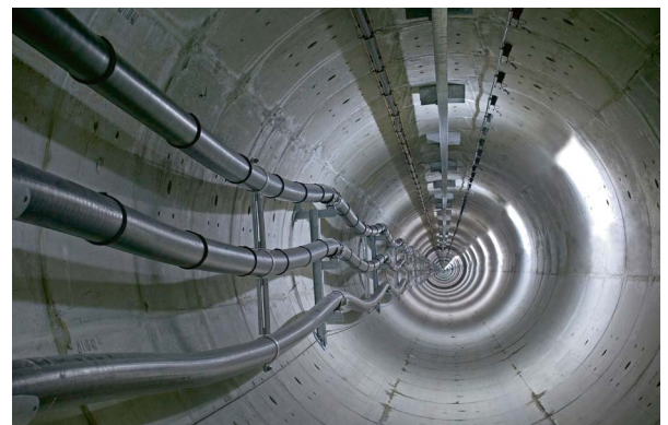
XLPE cables installed in a deep bore tunnel
