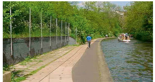
275kV cables installed in surface troughs along tow path
