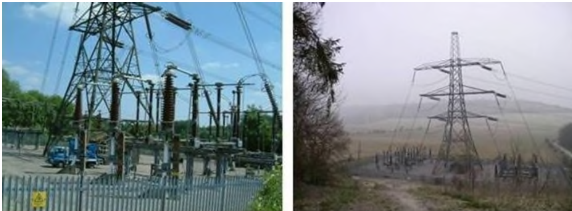
Figure C.5: Cable Sealing End Compounds
