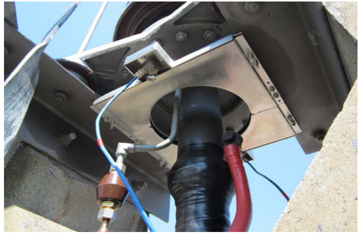
Rogowski-coil installed at Pitsmoor 275kV Substation Cable Sealing End
