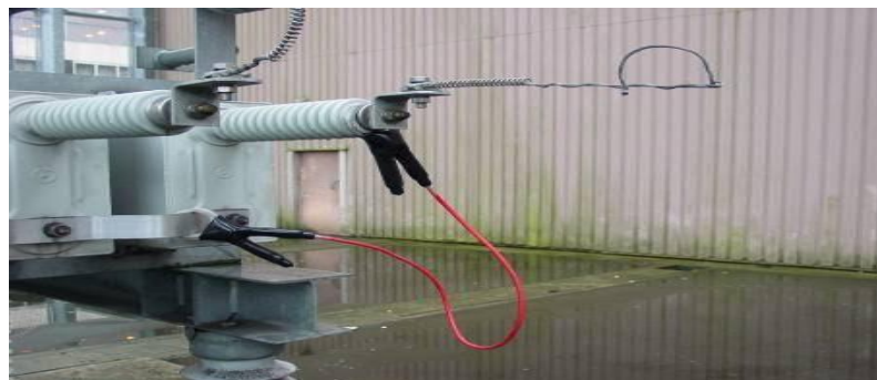
Figure 8.3A – Applying the Clip-on Short-Circuiting Lead
