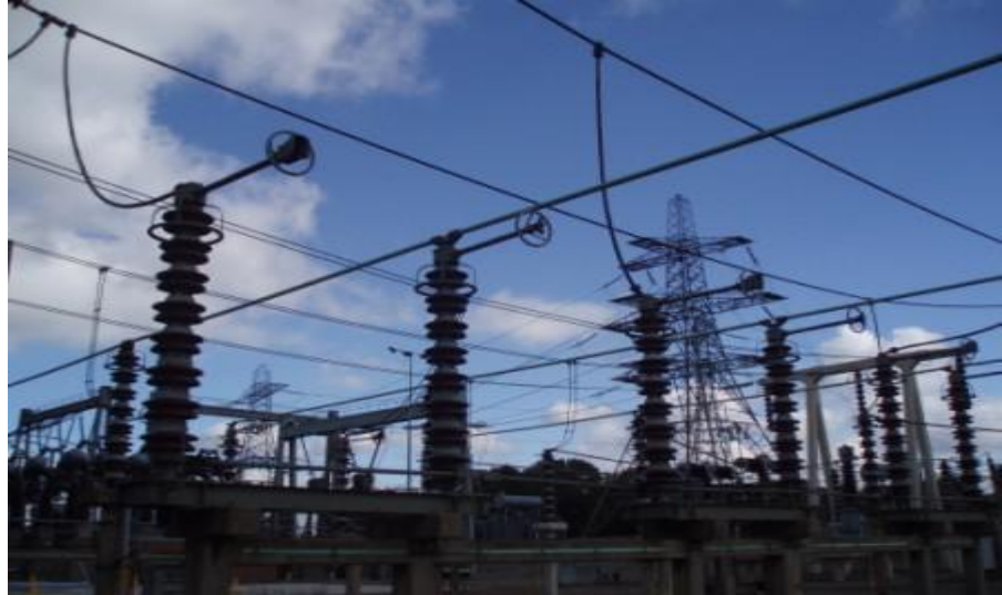
Figure 8.1A – End Rotating Post Busbar Isolators Arranged in Tandem
