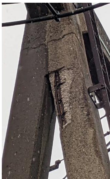
Image 2: Reinforced Concrete Support Structure Defect
