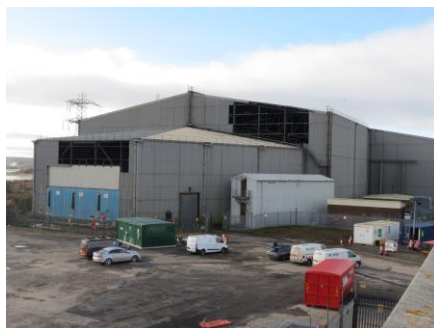
Image 3: Missing cladding at Blyth Substation
