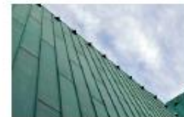
D Painted copper colour coated vertical cladding to rear (north) elevation and roof
