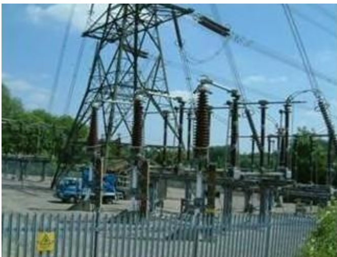
Image D.5 Cable Sealing End Compounds
