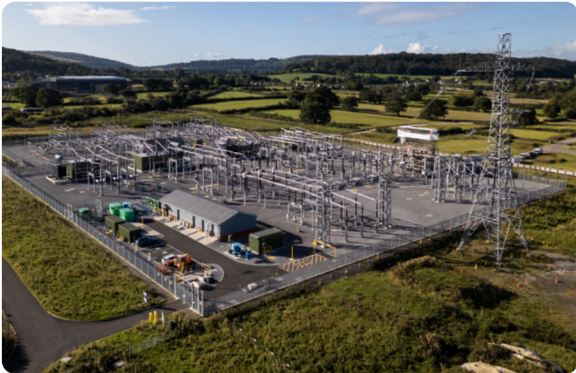
Figure 11: Example of a 400 kV substation for illustrative purposes only
