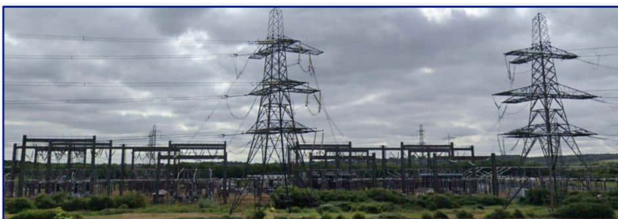
Image 4.4 Illustrative example of a typical AIS substation
