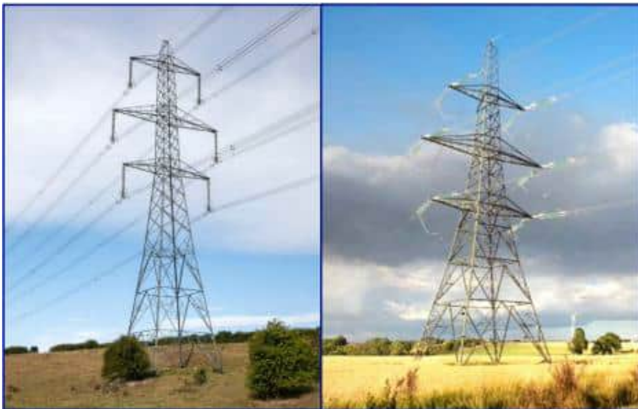
Image 4.2 Suspension tower (left) and Angle tower (right)
