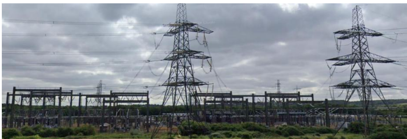
Image 4.5 Illustrative example of a typical AIS substation
