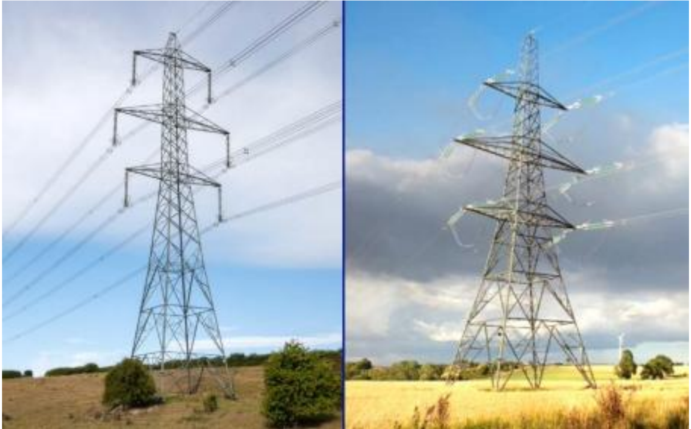
Image 4.2 Suspension tower (left) and tension tower (right)
