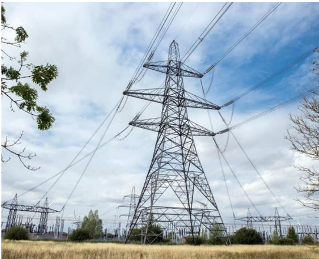
Image 4.3 Typical terminal pylon
