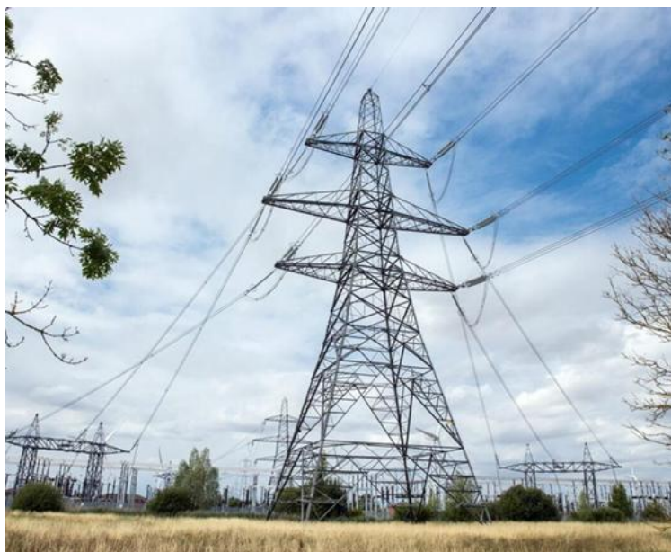
Image 4.3 Typical terminal lattice pylon
