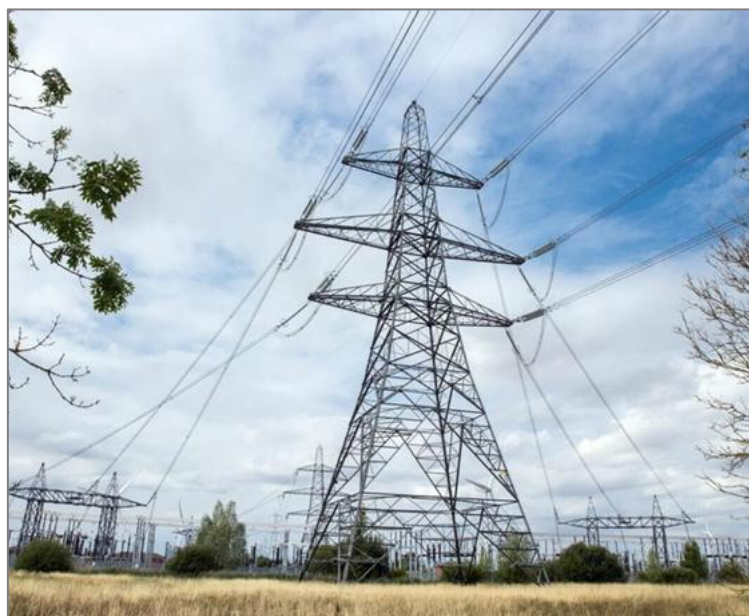
Image 4.3 Typical terminal lattice pylon
