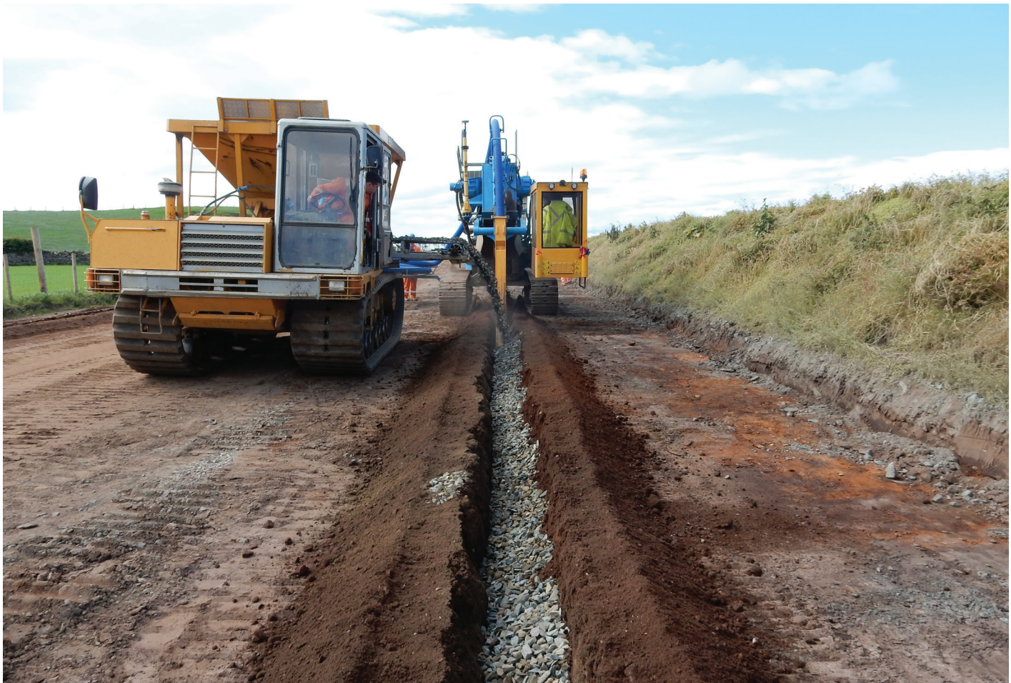
Example installation of pre-construction drainage system along High Voltage Direct Current project
