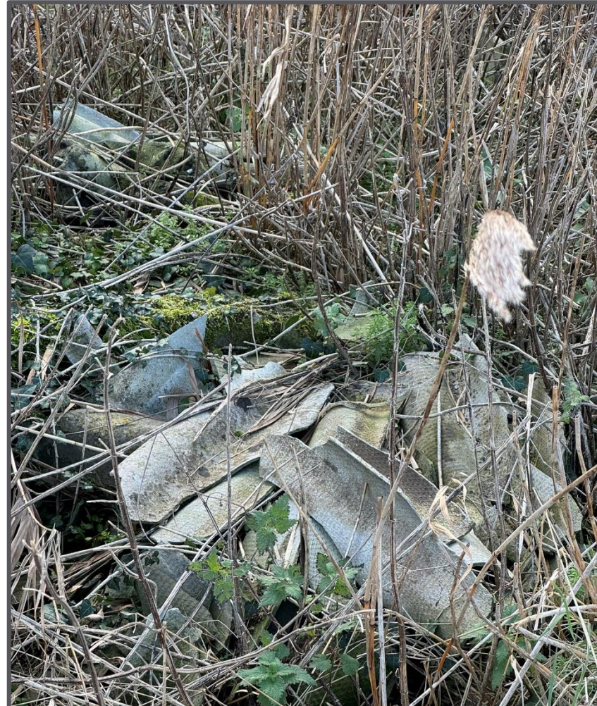
4e: Close up view of roof tiles noted (potential asbestos) (looking south).
