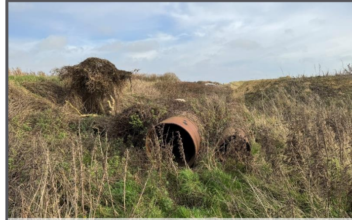
3f: View east of overgrown (disconnected) pipe infrastructure.
