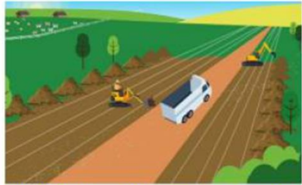
Step 2 The topsoil is carefully removed and stored separately alongside the trenches so it can be put back after the work is complete
