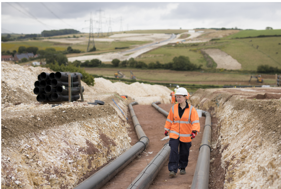
An example of undergrounding work at our Visual Impact Provision project in Dorset, UK
