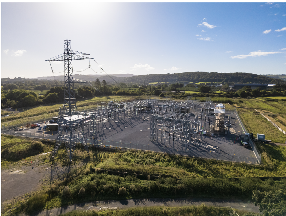
Sandford substation, part of the Hinkley connection project, UK
