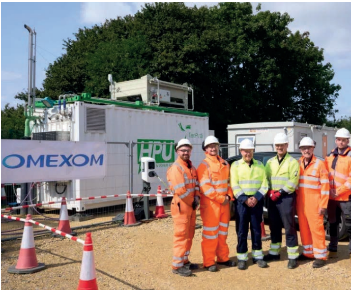
Powering the site
