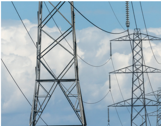
A 400 kV overhead line
