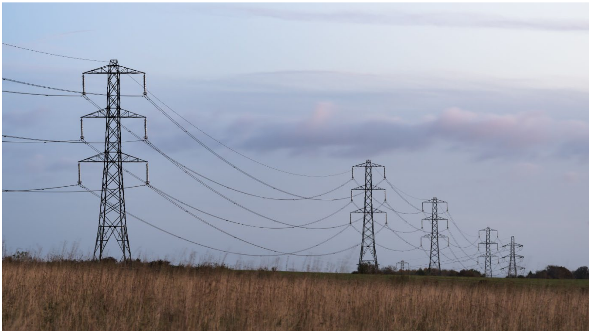
Figure 21: Existing ZF Overhead Line
