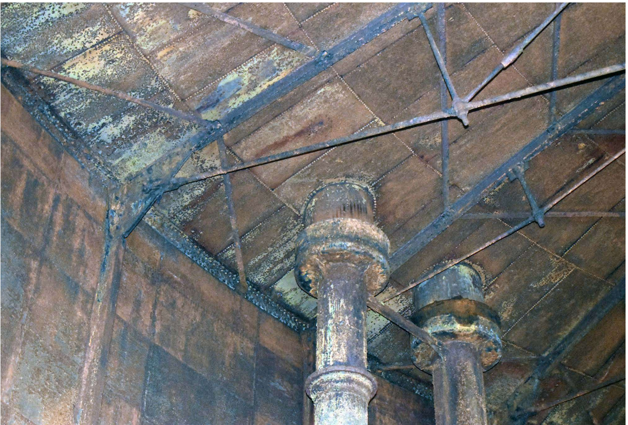
Plate 98: Head of inlet/outlet pipes
