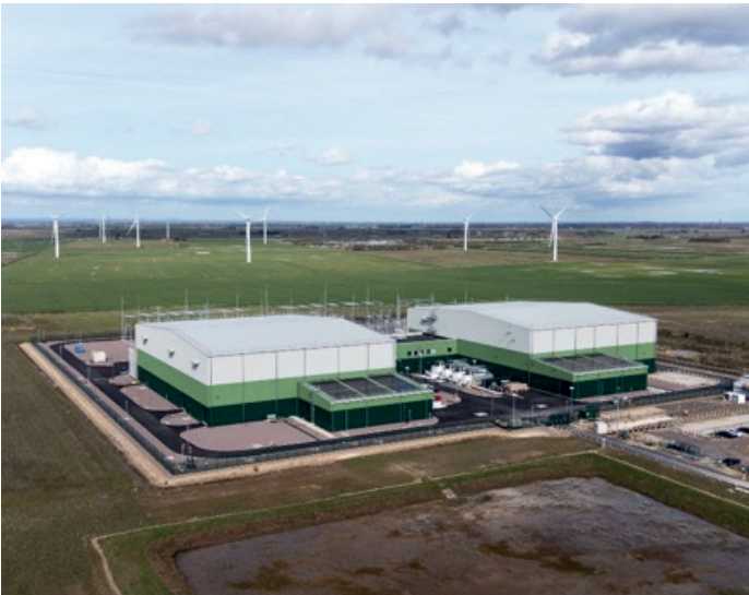
Figure 6 – National Grid Venture's Viking Link converter station, which illustrates what the EGL 3 and EGL 4 converter stations could look like
