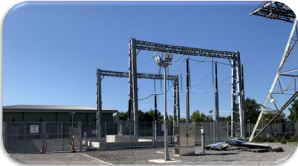
231kV 1-ph voltage capability
