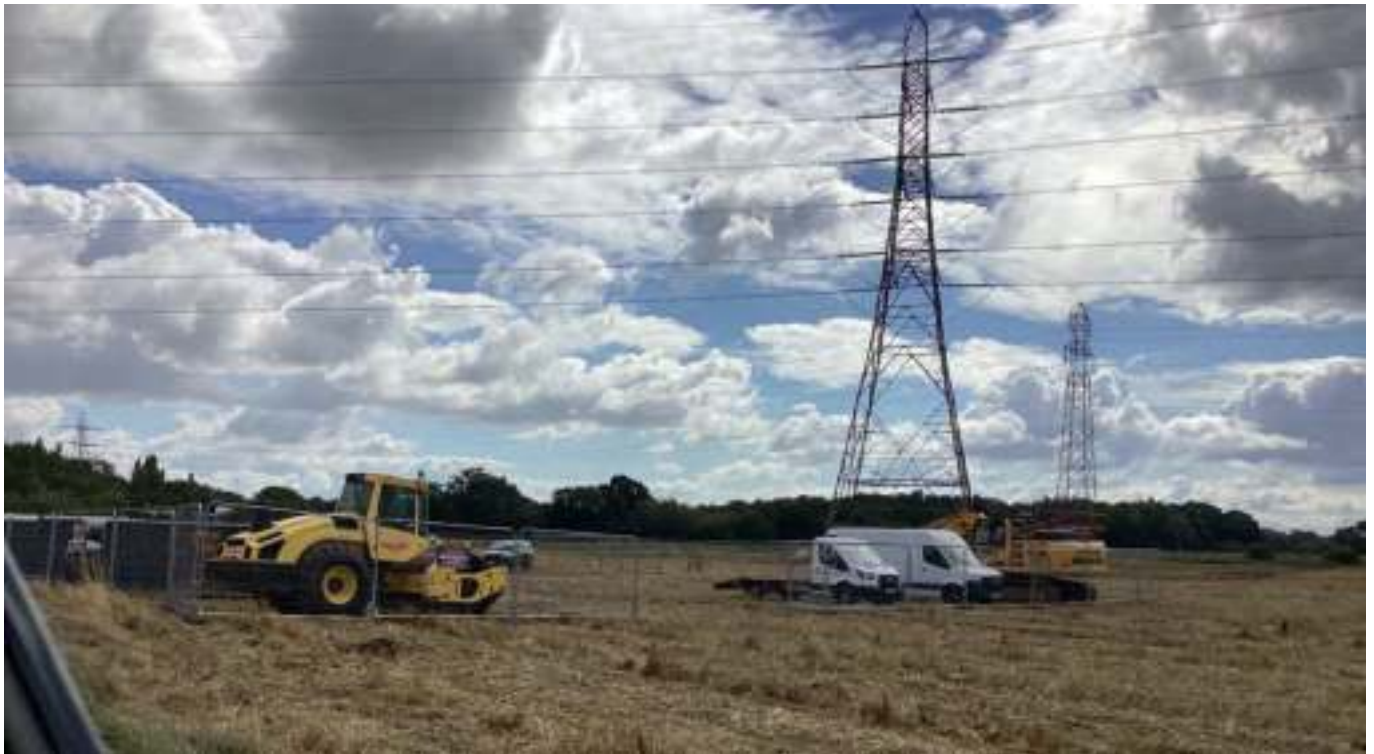
Plate 278: External company compound with vehicles and plant in crop field with pylons and overhead lines, looking east.
