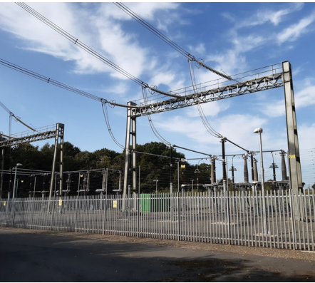
Cable sealing end compound
