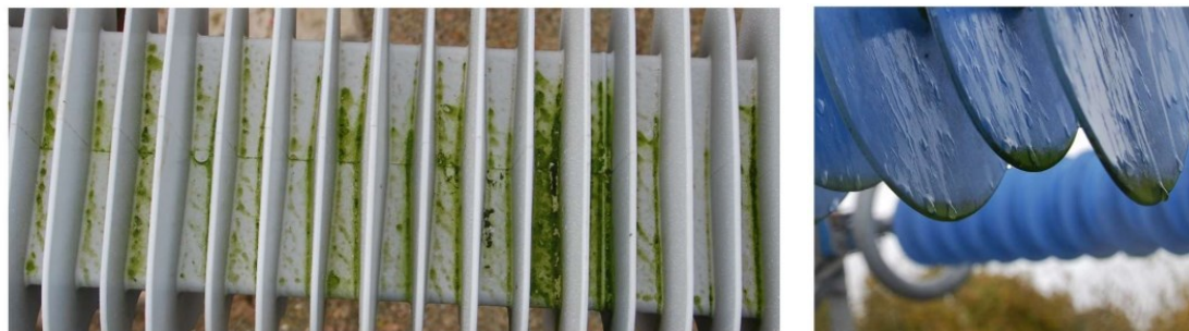
Figure 32 – Images showing the level of algae growth after 35 months in service.
