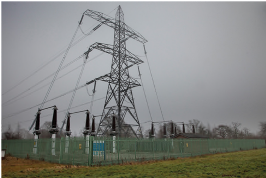
Figure 5.6 An operational sealing end compound
