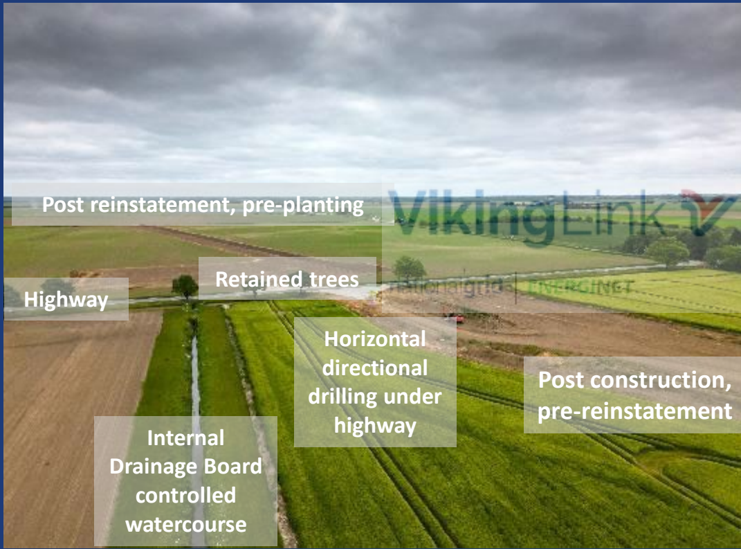
Agricultural land along cable working area post - construction (below highway) and post-reinstatement (above highway) with crops to be seeded by the landowner during the next planting season.
