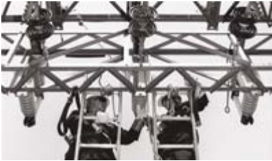
Left National Grid USA's training centre in Massachusetts houses more than a dozen classrooms, conference rooms and hands-on skills training areas. The centre includes outdoor 'laboratories' where students train on overhead and underground electricity distribution equipment such as transformers, poles and a working substation.
