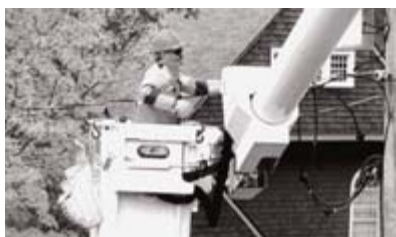
Left National Grid USA performs regular maintenance on a 72,000-mile distribution network in order to maintain reliable electricity services to 3.2 million customers in the northeastern US.
