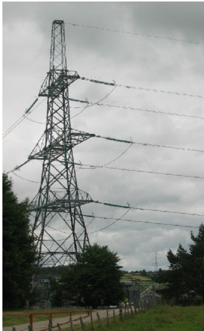
Typical example of a Terminal Tower
