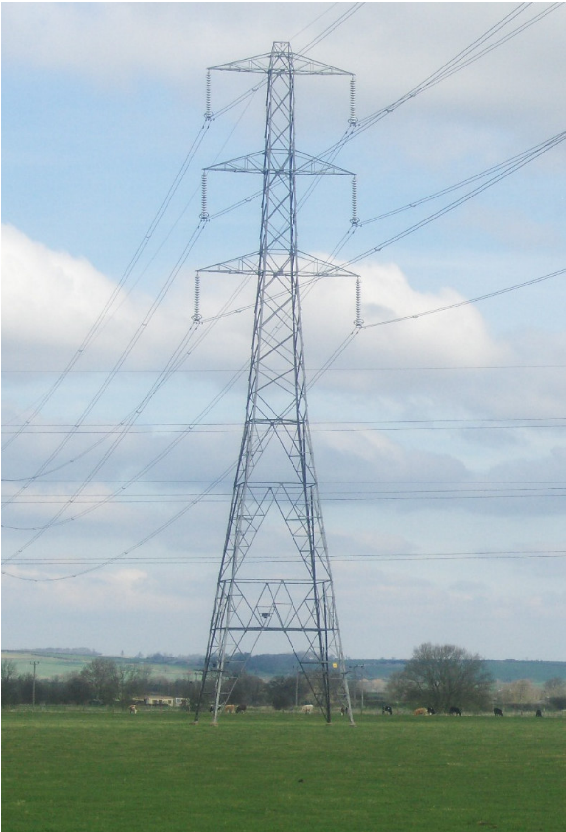
Typical example of a Suspension Tower
