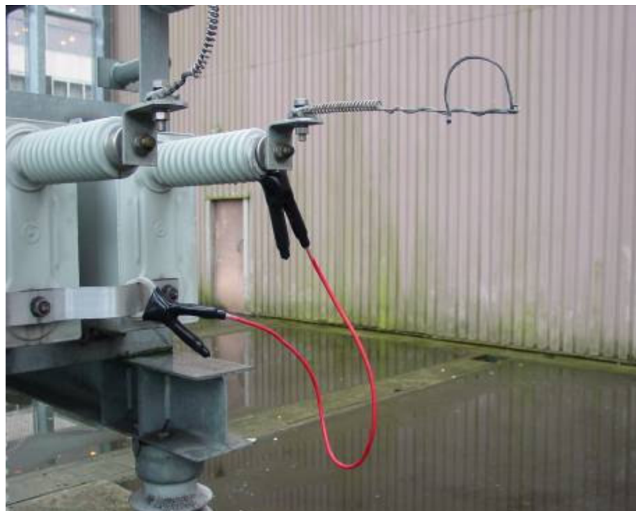
Figure 6.3A – Applying the Clip-on Short Circuiting Lead
